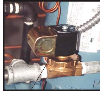
Typical water make-up solenoid valve
