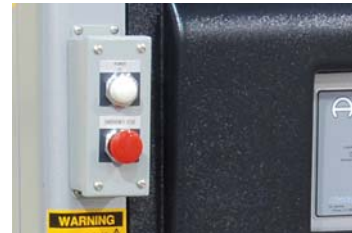
Emergency stop button. Shown with Power On light.
