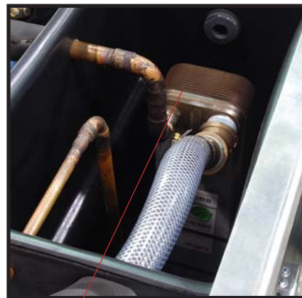
Typical Evaporator in Reservoir
