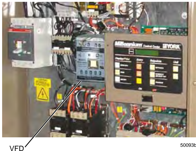
FIGURE 45 - TYPICAL VFD LOCATION
