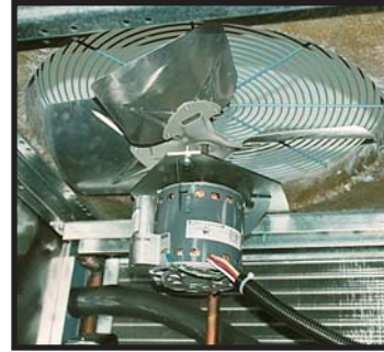
Typical fan assembly
