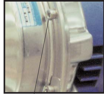
Typical pump casing bolt
