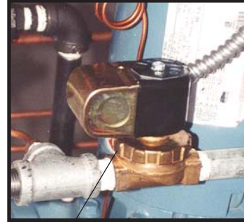
Typical water make-up solenoid valve
