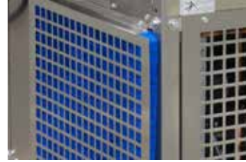
Typical Condenser Screen.
