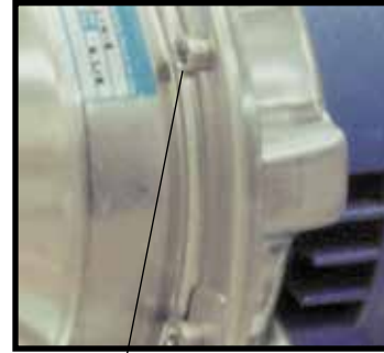
Typical pump casing bolt
