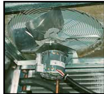
Typical fan assembly
