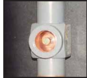
Refrigerant sight glass Figure 7.2D
