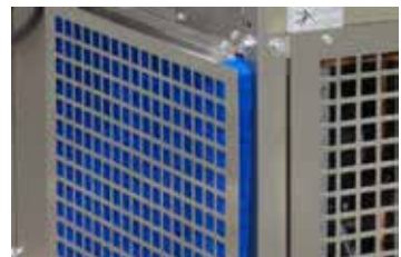
Typical Condenser Screen.
