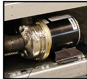
Pump motor Figure 5.5B
